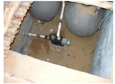
Surface Pump for Pool Circulation
