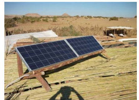
PV system for Steca DC Refrigerator
